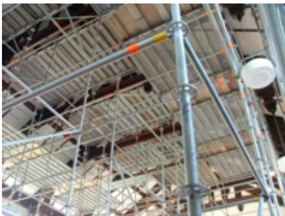
The Hall is a forest of scaffolding and platforms as the ceiling and walls were repainted. 2006.
